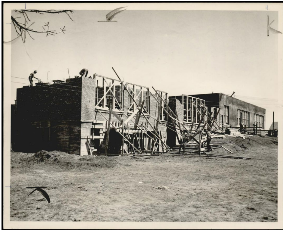
Construction photograph used for a story in the Oklahoma Times newspaper. Caption: "Construction work on the $93,121 addition to Creston Hills school, 2240 NE 19, provides additional playtime interest for pupils during recreation periods, as masons raise the addition on the west side of the old building." Oklahoma Times, Oklahoma City, Oklahoma, April 5, 1949
